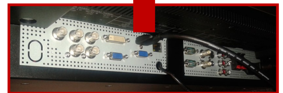
The cable and power source connections to the NEC screens are accessible underneath the screen
